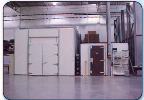
EMI Semi Anechoic Chamber and Shielded Control Room
